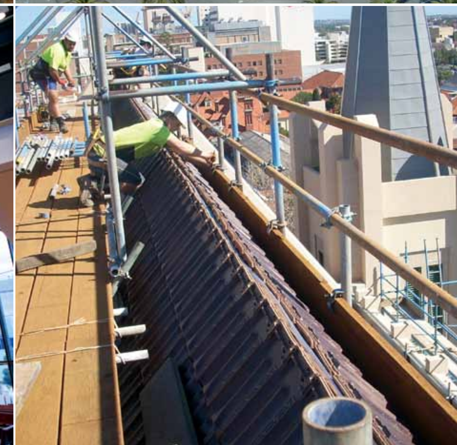
Photography: Main images by Ron Tan Photography, courtesy Roman Catholic Archbishop of Perth, construction image by John Rawlins.
